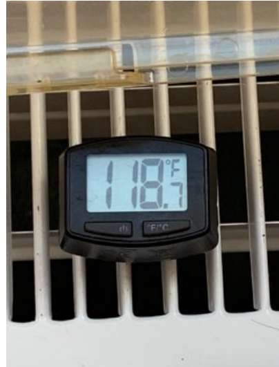
Supply air temperature from furnace.
