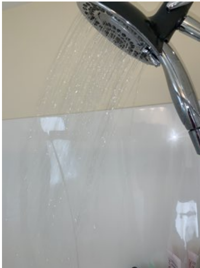
Bedroom bathroom shower
