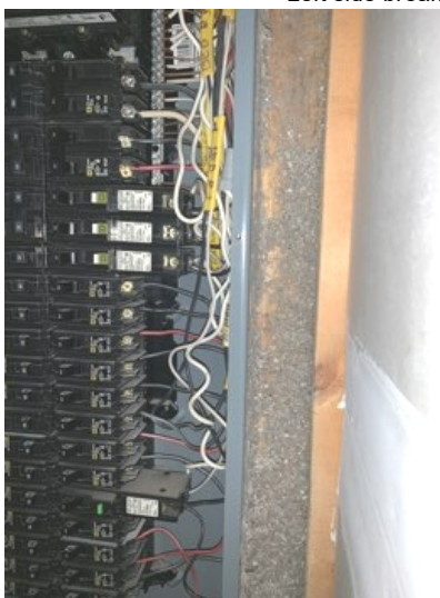
Right side breakers and neutral bus bar: no deficiencies observed.
