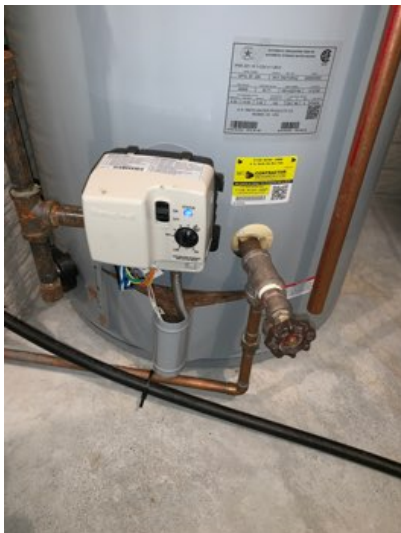
Base of water heater: no leaks, corrosion or damage observed
