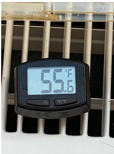
Supply air temperature from A/C unit
