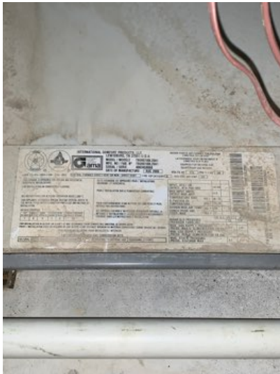
Furnace data plate with information and specifications.
