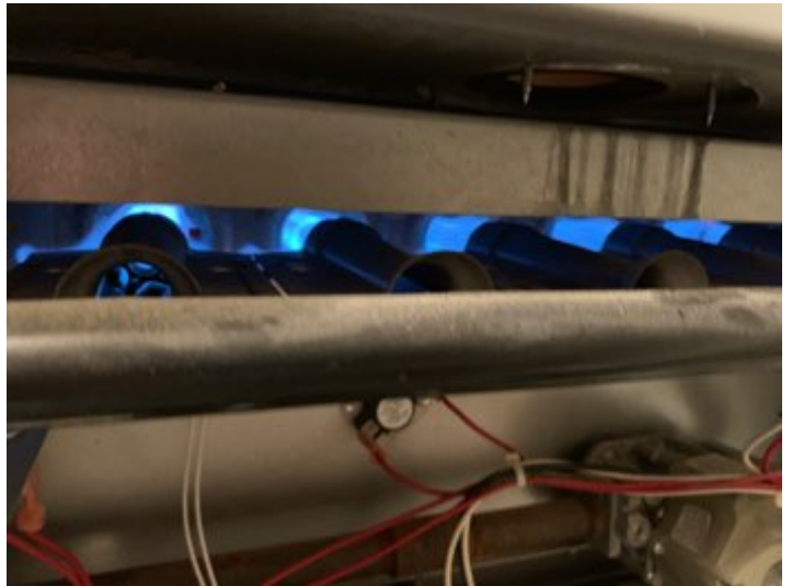
Flames burn bright blue indicating proper fuel combustion.
