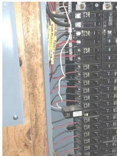
Left side breakers and neutral bus bar: no deficiencies observed.
