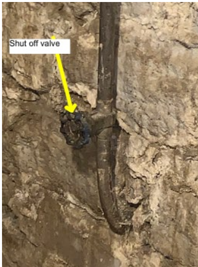
Water supply and whole house shut off valve.
