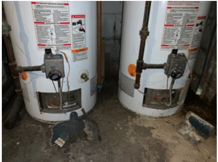
Bases of water heaters: no leaks, corrosion or damage observed
