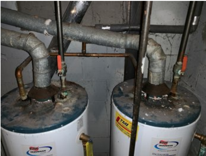
Tops of water heaters: no leaks, corrosion or damage observed
