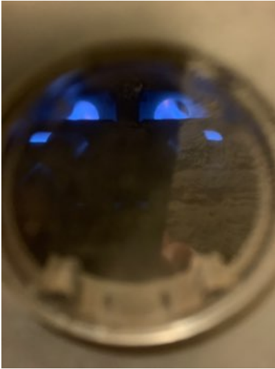
Flames burn bright blue indicating proper fuel combustion (basement unit).
