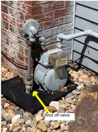
Gas supply, meter, and whole house shut off valve.
