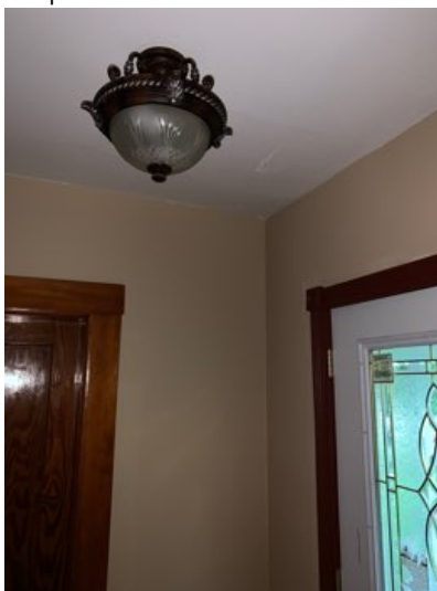
REPAIR- The side door interior entry light fixture was not working. Recommend contacting a certified electrical contractor to assess and repair as needed.
