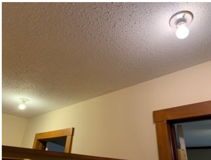
REPAIR - Multiple closet light fixtures were an exposed light bulb type. This is less safe. Recommend contacting a licensed electrical contractor to assess and repair as needed.
