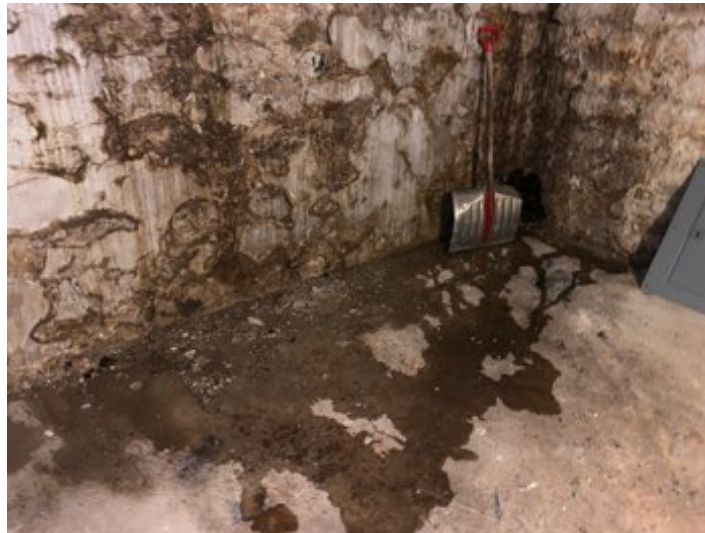
REPAIR- Water/moisture intrusion observed. Water may damage building finishes and structural components as well as aid in the growth of mold. Recommend contacting an appropriate reputable contractor to assess and repair as needed.
