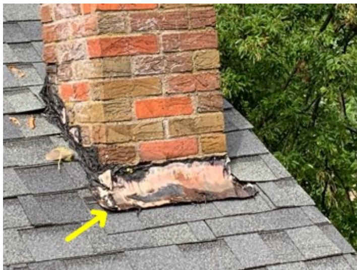
REPAIR- The chimney flashing appears to be insufficient. This may lead to water entering the building resulting in damage to the structure and finishes as well as aid in the growth of mold. Recommend contacting a licensed roofing contractor to assess and repair as needed.
