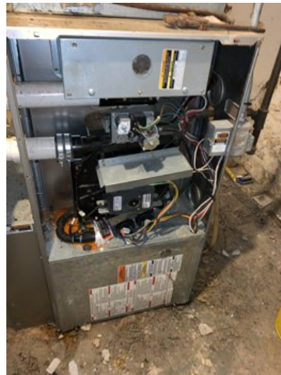
Interior of furnace cabinet: no deficiencies observed.
