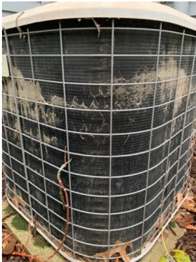
MAINTENANCE - The exterior coil was dirty and needs cleaned. Keeping the coil clean will help with efficiency and help prevent premature failure. Recommend cleaning the coil upon possession of the home and annually thereafter.
