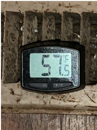
Supply air temperature from Amana A/C unit
