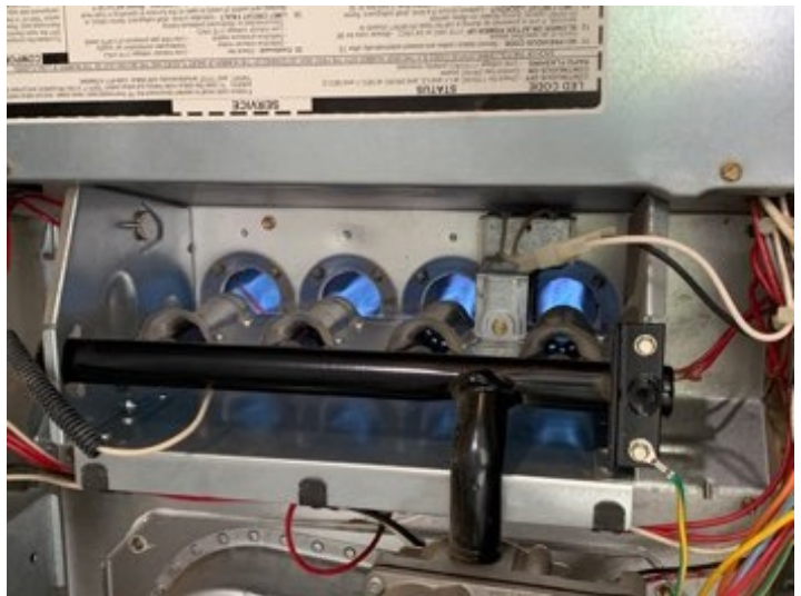
Flames burn bright blue indicating proper fuel combustion (garage unit).
