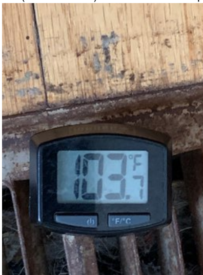
Supply air temperature from basement furnace.
