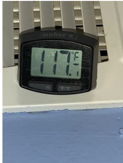
Supply air temperature from furnace.
